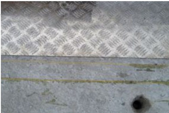
Glued fiber optic on Bridge
